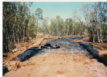
Temporary roads are underlain by filter cloth so as to reduce impacts to habitat and facilitate road removal
